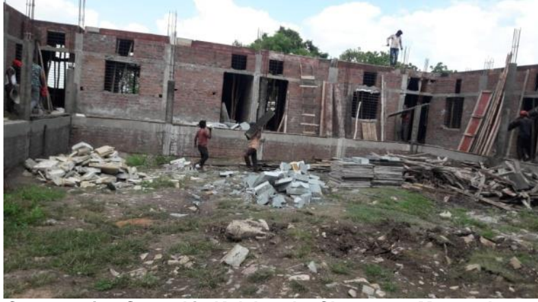
New School Building Construction Started in Kulakunda ,Chamanur, Muguta by our Advocacy
